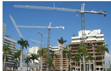
Tower cranes use extra components as the height of the building increases. Keeping track demands effective systems.
