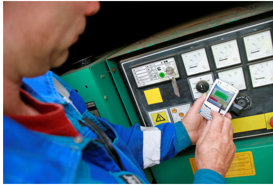
An RFID tag identifies on-site plant and prompts for required maintenance.
